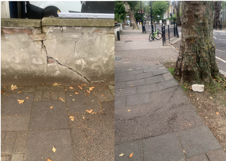
The roots of a London plane tree crack an adjacent wall (left) after meandering below the paved sidewalk (right). Photos: Aaron Bradshaw, 2023.
